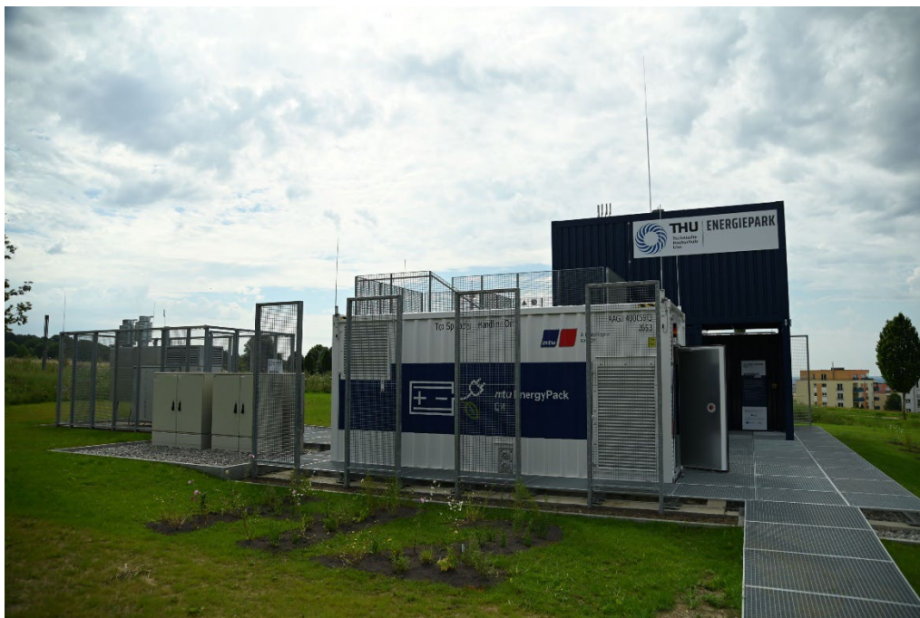
Foto 3: THU-Energiepark am Eselsberg in Ulm
